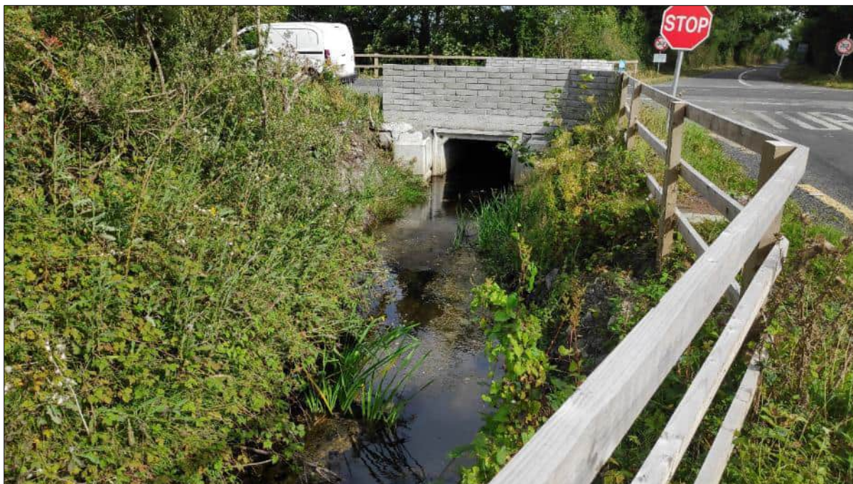
Plate 4.17 Representative image of site B12 on the Feeghroe River at Five Roads Cross, August 2022 (facing upstream to upgraded box culvert)
